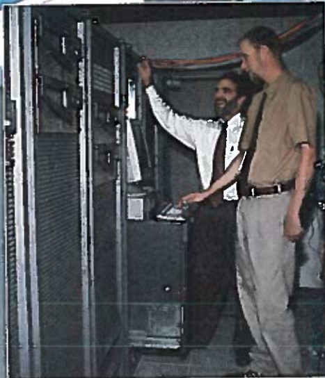
The District Office currently houses the Wide Area Network System.
